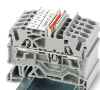
Orient the staggered jumpers' red stripes on the inside. Insert the staggered jumper and push down until it hits the backstop.
